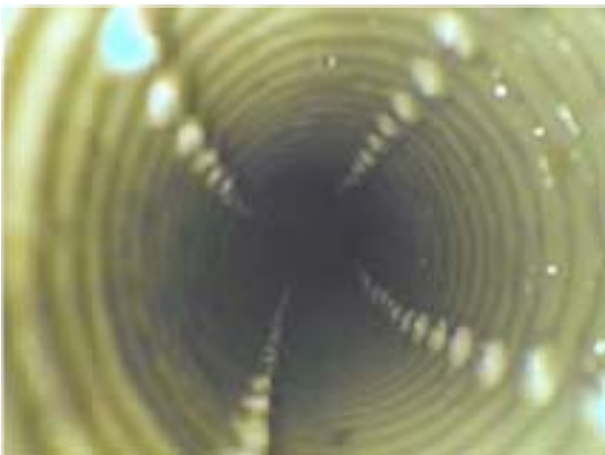
Figure 7. Mini-pipe free of damage
