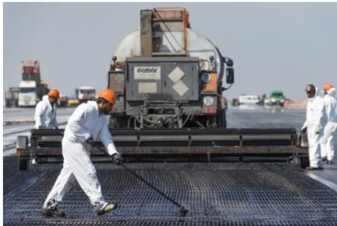
Figure 2. Laying of a reinforcement geosynthetics on runway 2 of Paris CDG airport in 2016. Picture courtesy of Colas
