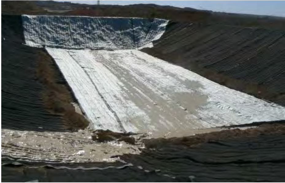
Figure 14: Slurry dewatering facility (photo courtesy Afitex-Textel)
